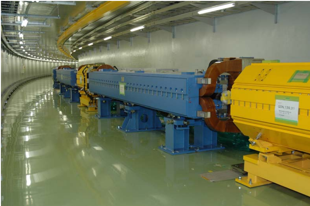
Dipoles and quadrupoles in Arc-C
